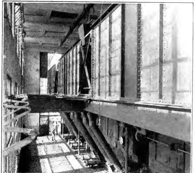
INTERIOR OF BOILER ROOM WITH BUCKET UNLOADING AT MOUTH OF SELF-FEEDING HOPPER
